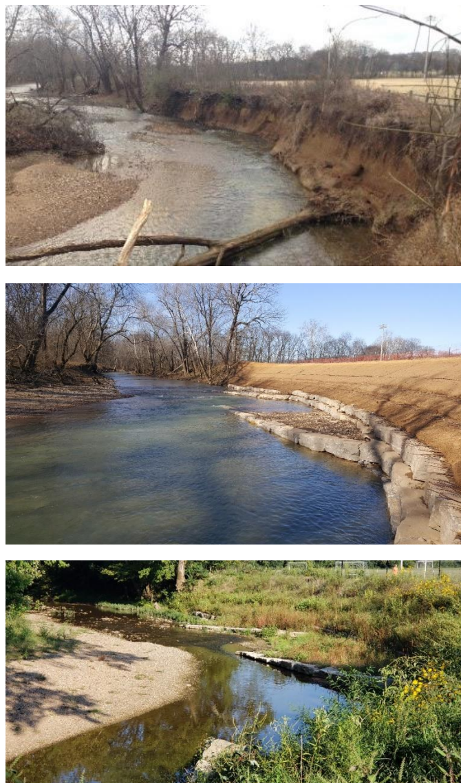
Figure 7. Before, immediately after, and one year following construction of a vegetated soil lift with boulder toe.
