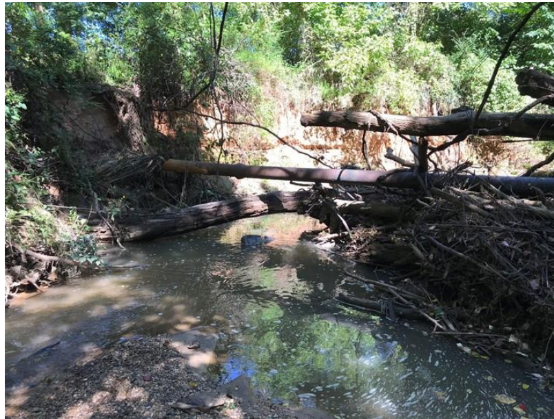
Figure 4. An aerial sewer line cross on Duharts Creek that is catching large amounts of woody debris.
