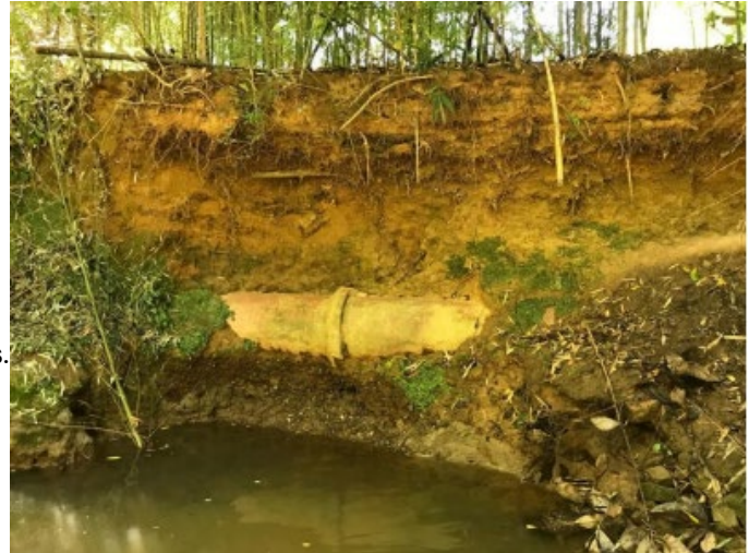
Image 1. Exposed underground sewer pipe in Duhart's Creek at a point of active erosion.
