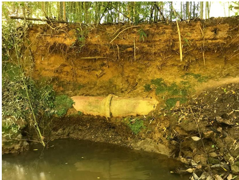
Figure 6. Photo of exposed underground sewer pipe in Duharts Creek at a point of active erosion.
