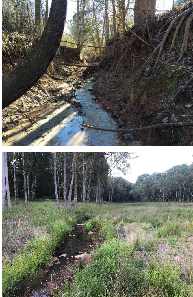
Figure 8. Before (above) and less than one year (below) after construction showing a stream with restored floodplain.
