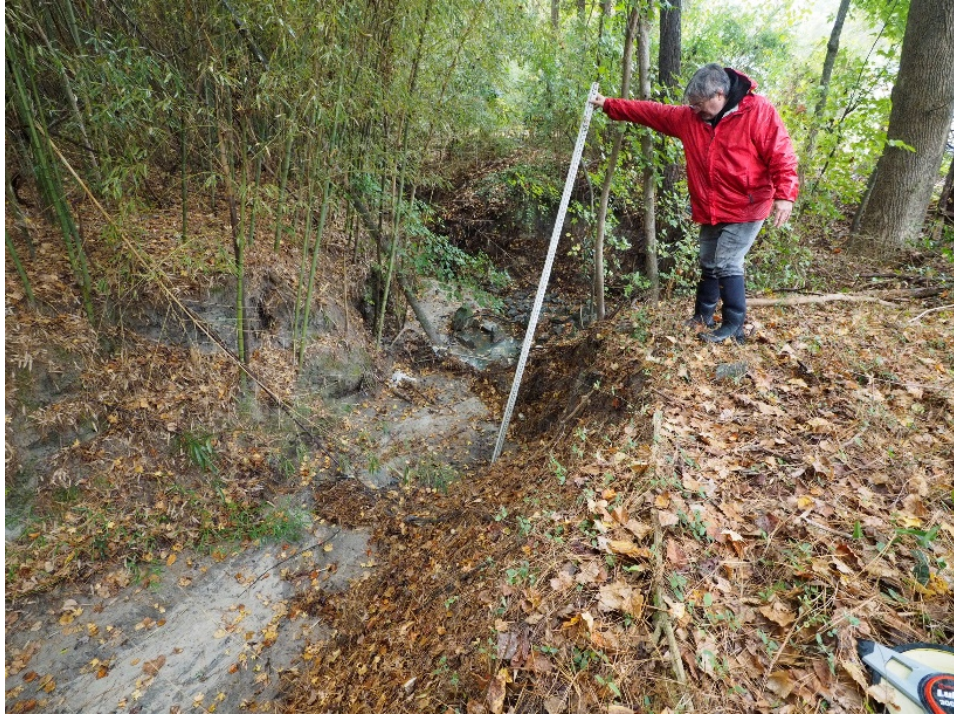
Figure 1. Typical channel erosion, 9 feet deep, 14 feet wide.
