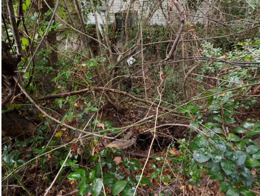
Figure 5. Exposed electric service casing pipe (foreground) and threatened structure (background).
