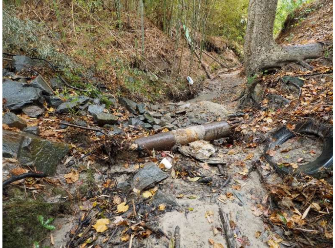
Figure 2. Exposed Sewer Asbestos Cement Pipe Crossing
