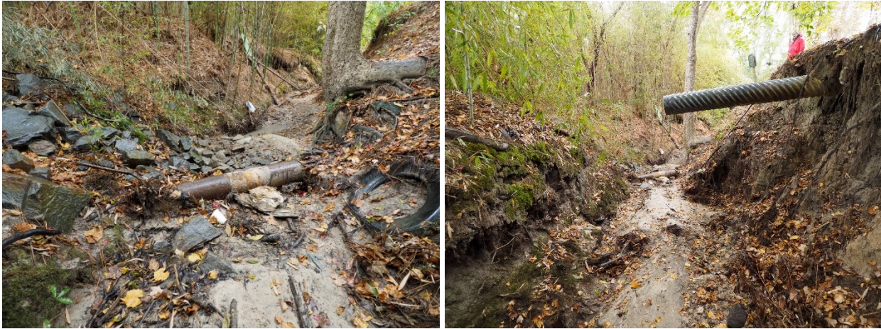
Figures 3a & 3b. Exposed sewer line and SW discharge upstream of sewer line.
