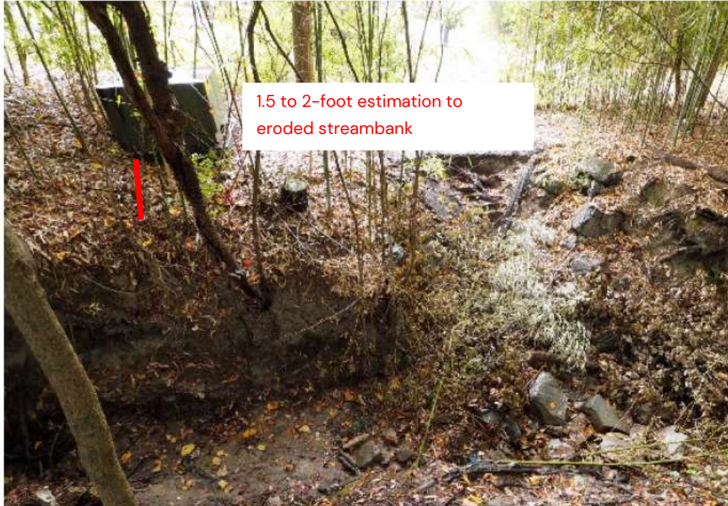
Figure 4. Second transformer box near eroded streambank
