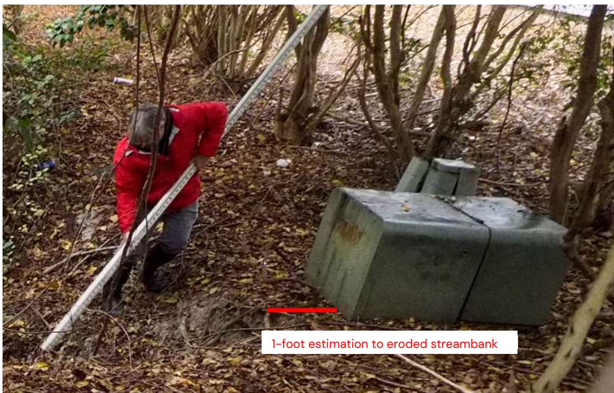
Figure 3. Transformer box near eroded streambank
