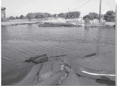
Road in Hatteras Village destroyed during Hurricane Isabel in 2003
