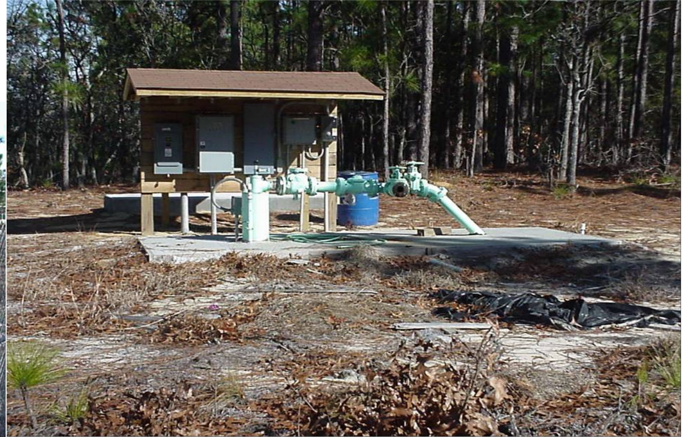
After a PA project written with 406/HM: The well site was relocated. Reconstruction of well head and controls above 100-year flood elevation. Area cleared to prevent any trees from falling on well head controls.
