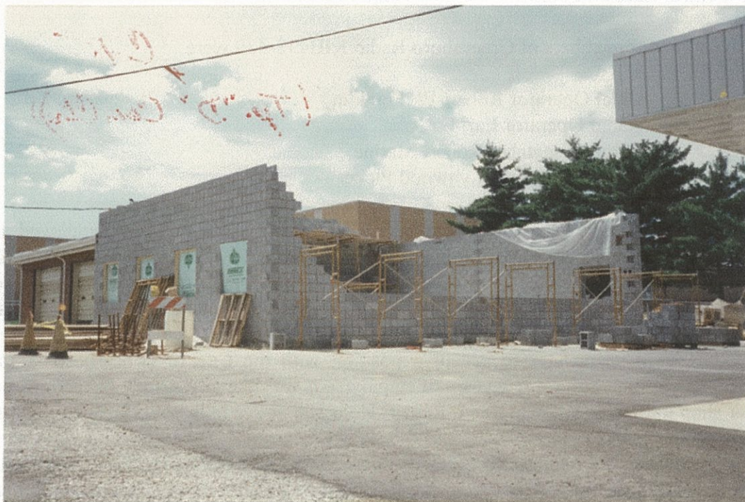
Top: Troop "D" Communications Center, new and first activated 1953. It was vacated by 1 May 1990 for the second home, shown being constructed in the bottom photo. The main entrance is to the far right, and the radio repair shop was located inside, to the far left end. The two story building to the right is that of Troop "D" Headquarters. Greensboro, NC. Photo taken 27 June 1995.
