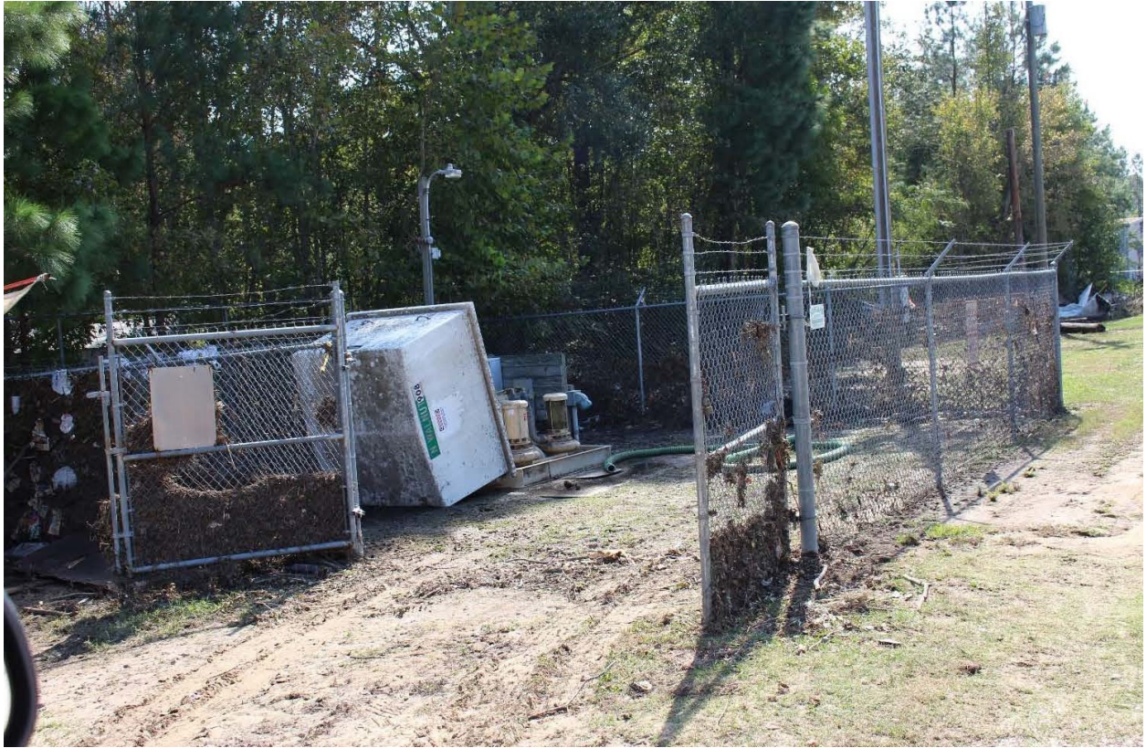
N. Walnut Street pump station site with leaves and debris in the fence that show the water level during hurricane flooding
