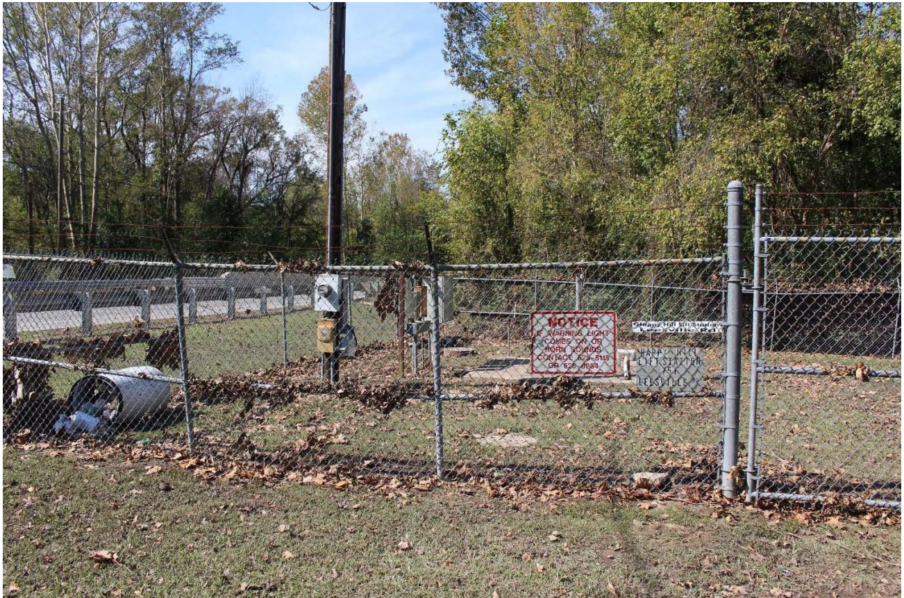
Happy Hill Pump Station – Leaves on the fence show that the pump station was thoroughly submerged during hurricane / Note location of utility pole for reference to previous photo
