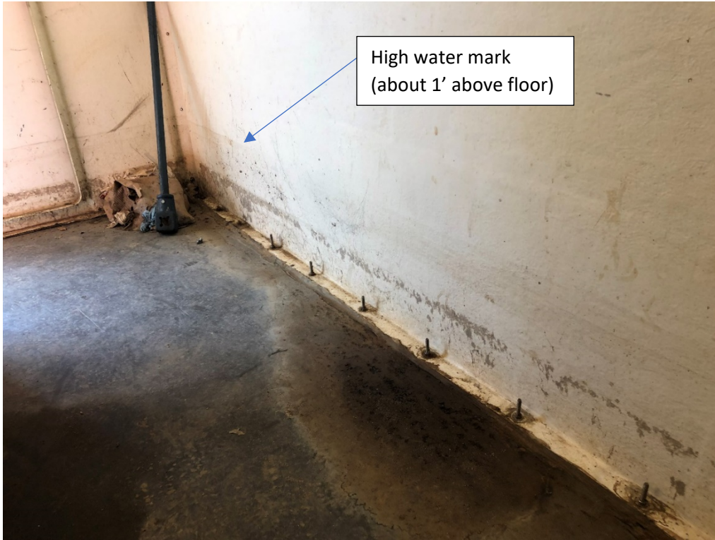
Inside of Pump Station Enclosure/Building – Showing Water Stains from November 12, 2020 Flooding
