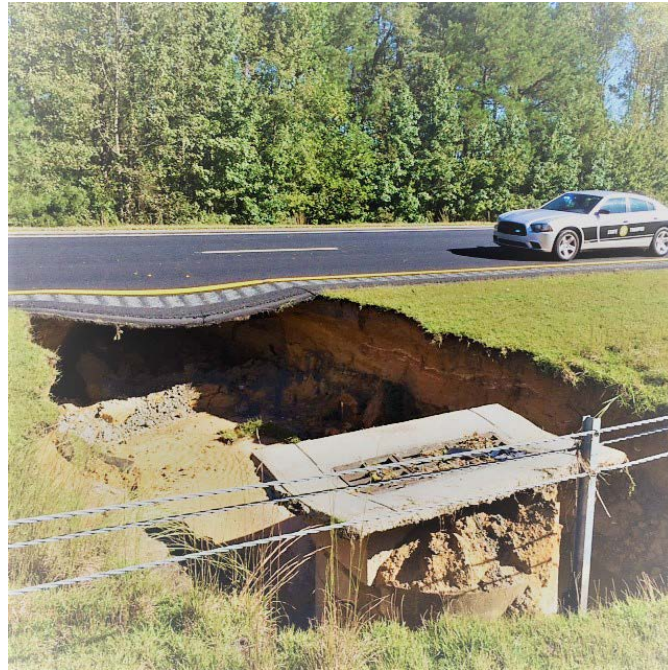
FIGURE 5.12: SINKHOLE IN NORTH CAROLINA
