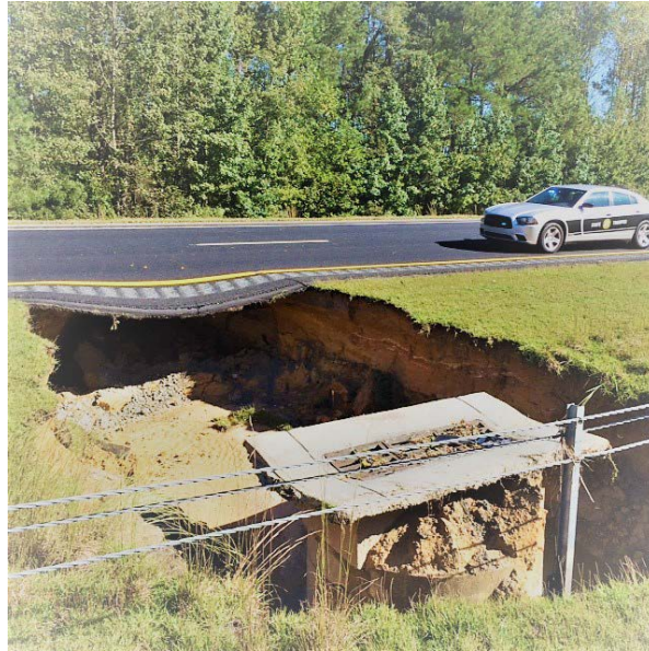
FIGURE 5.12: SINKHOLE IN NORTH CAROLINA
