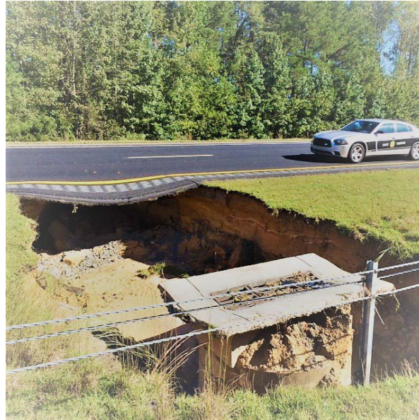
FIGURE 5.12: SINKHOLE IN NORTH CAROLINA
