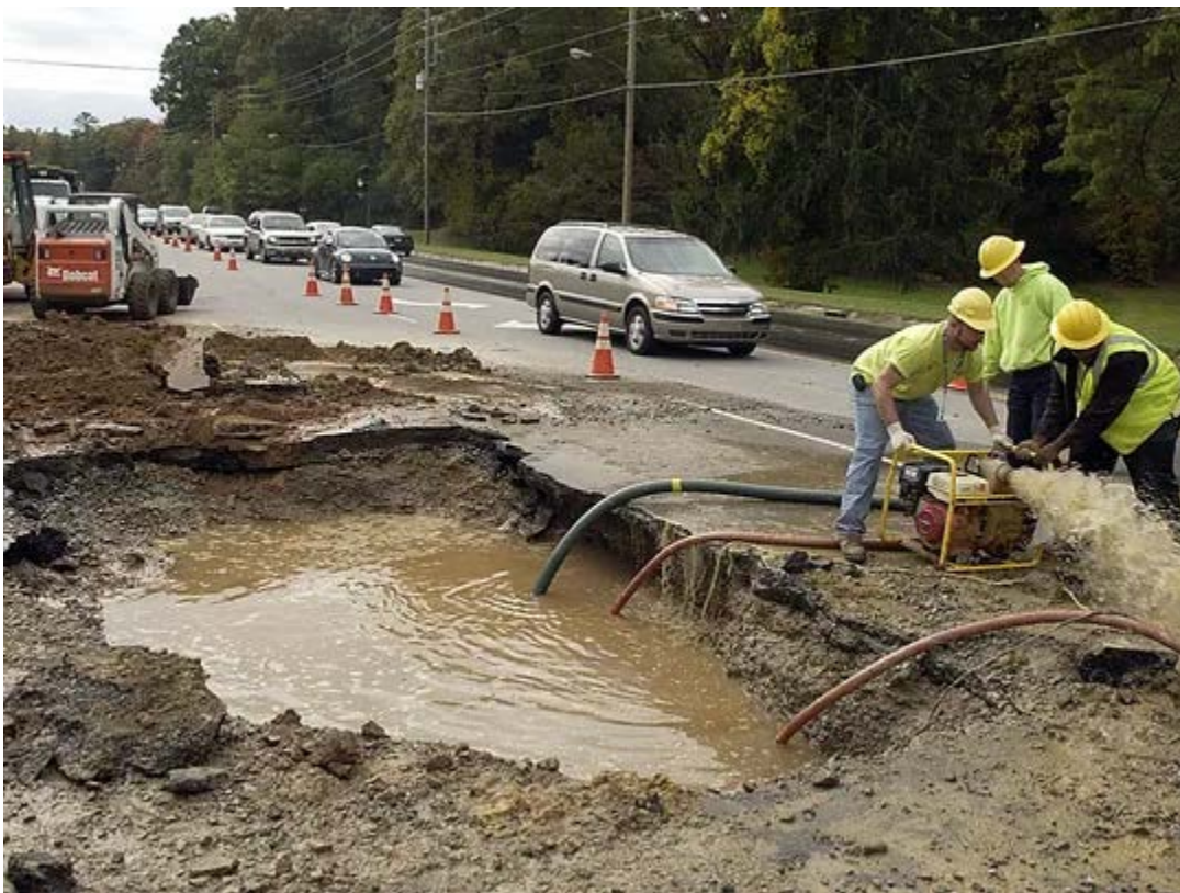
FIGURE C.11: SINKHOLE IN BUNCOMBE COUNTY
